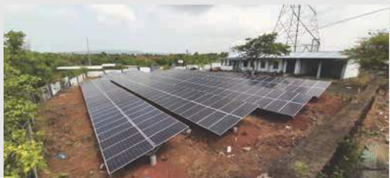
100kWp Solar power plant at 110kV KSEB Substation, Pazhayangadi, Kannur
