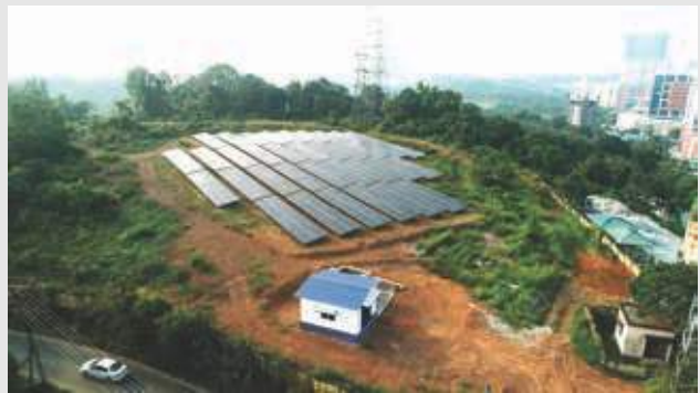
0.5 MWp Solar power plant at KSEB BDPP - Brahmapuram
